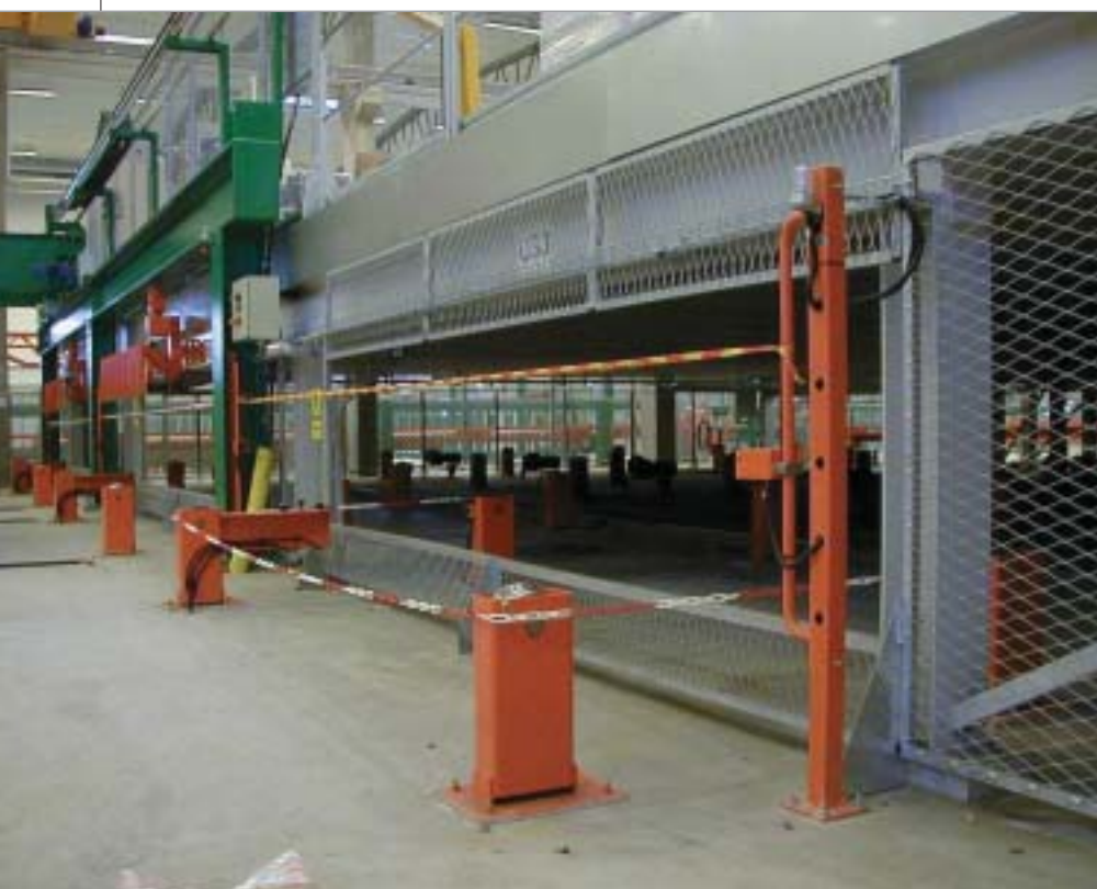
Pallets passing through – protected by light barriers
