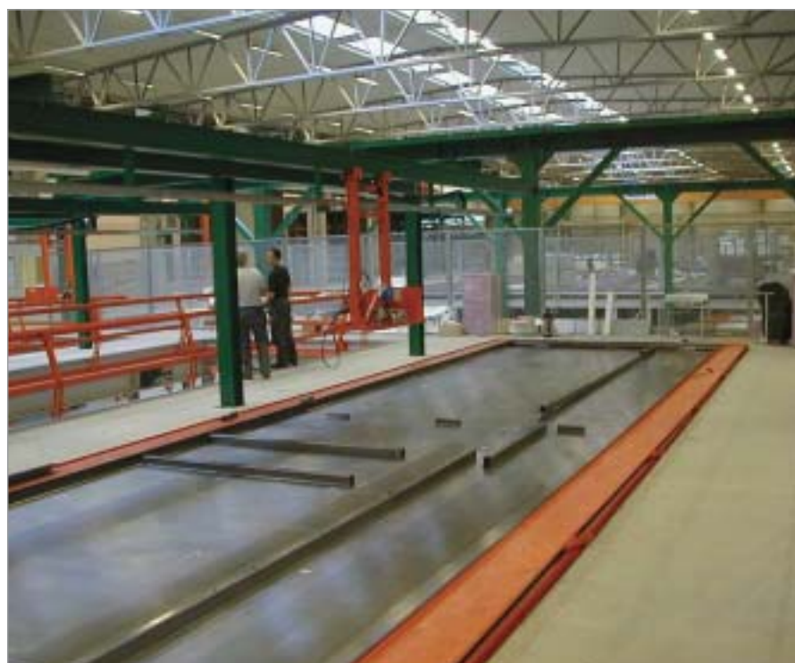
Manual shuttering stations
