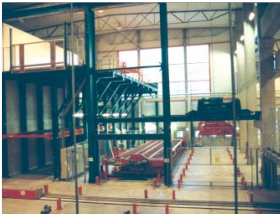
Additional rack with platform and double wall production
