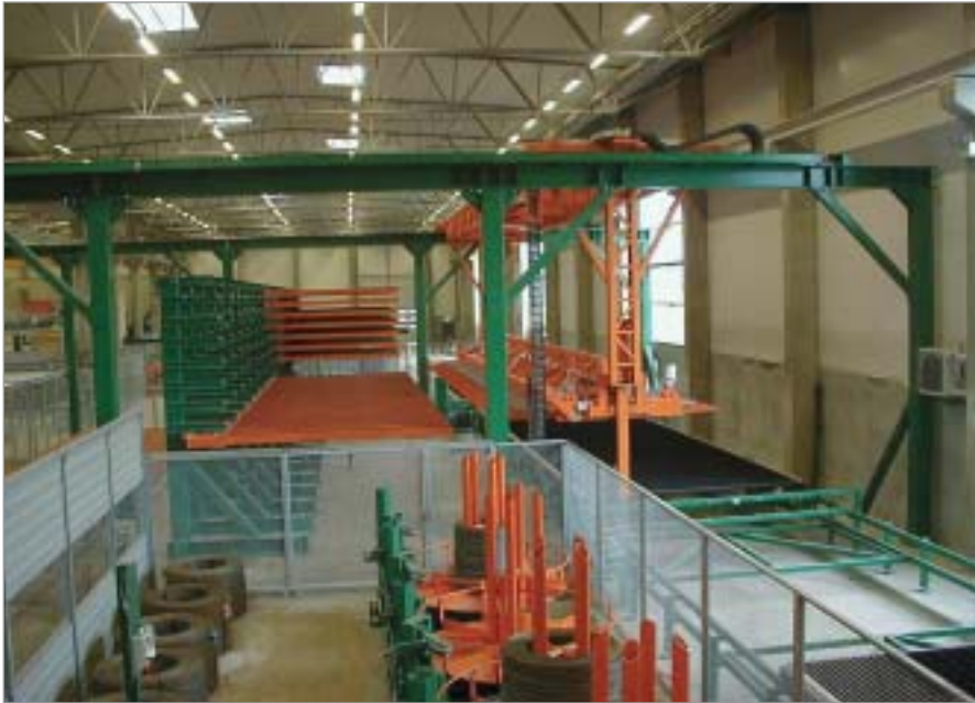
Mesh welding plant and reinforcement mesh store
