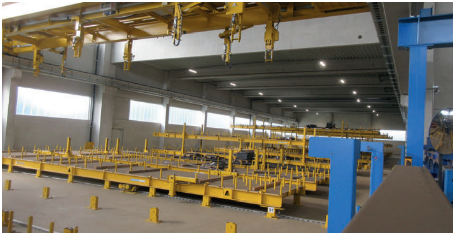
Automated storage collecting pallets
