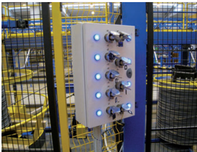
Fig. 41: Fortress mGard Access Key Exchange Panel
