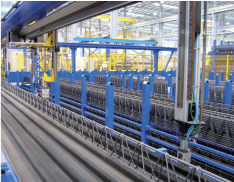
Fig. 33: Lattice Girder Active Store
