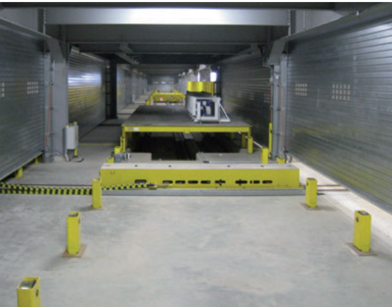
Fig. 18: Pallet and Central Transfer Car in Tunnel
