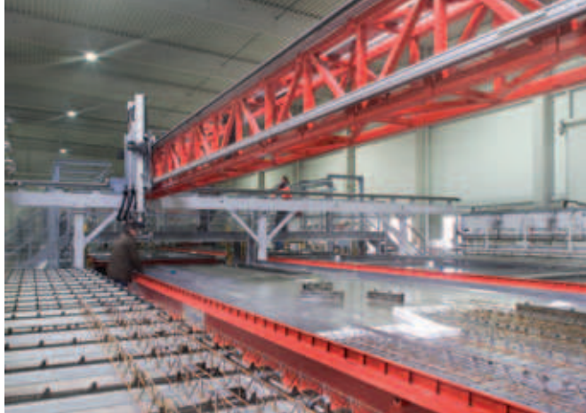
Picture of the double-line pallet guidance in the reinforcement robot area
