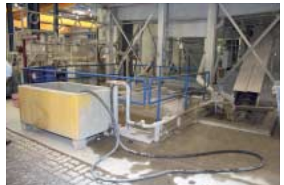
Fig. 5 The recycling plant for washing water and residual concrete.
