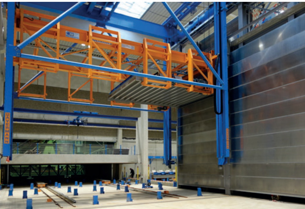
Storage and retrieval machine for hardening chamber feeding
